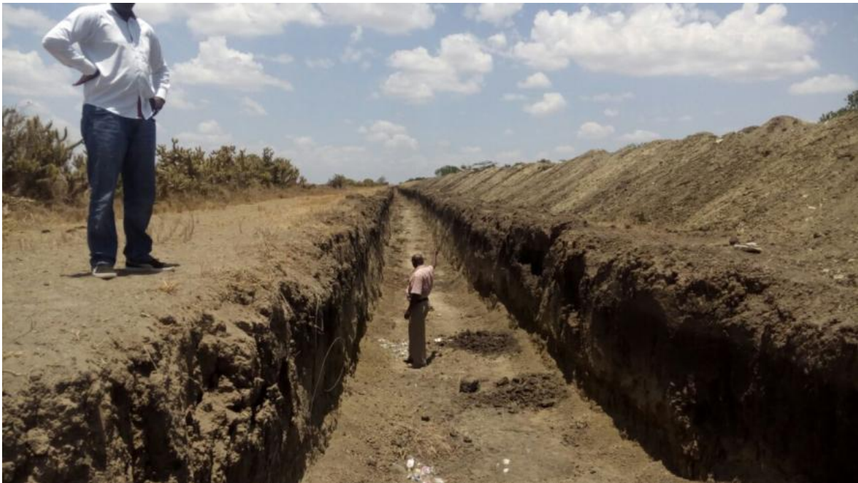
Plate 1: A section of the moat estimated total length of this section is about 16km where fence was destroyed by illegal grazers
